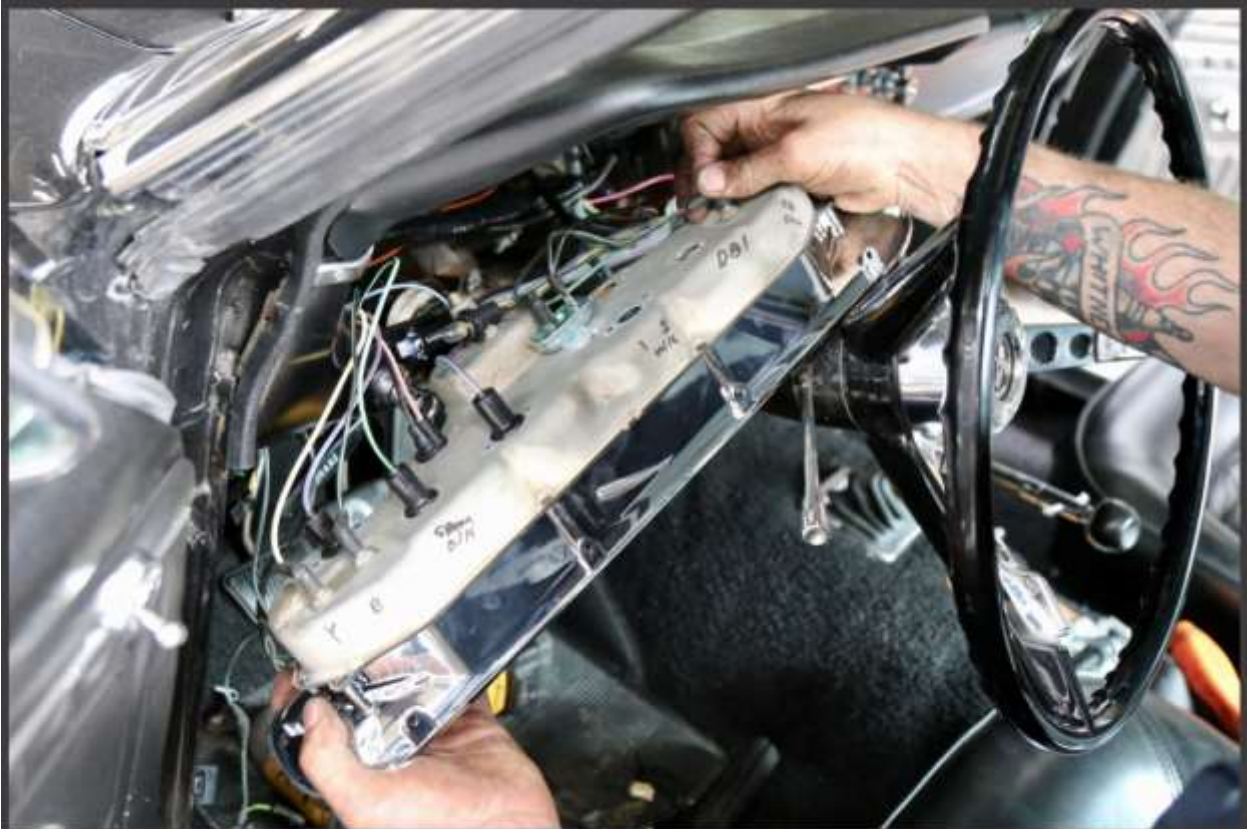
One end of a new speedometer cable and the appropriate gear were installed in the Toploader transmission before the gauge panel reassembly began. All the connections were made using the notes and wire color coding.
