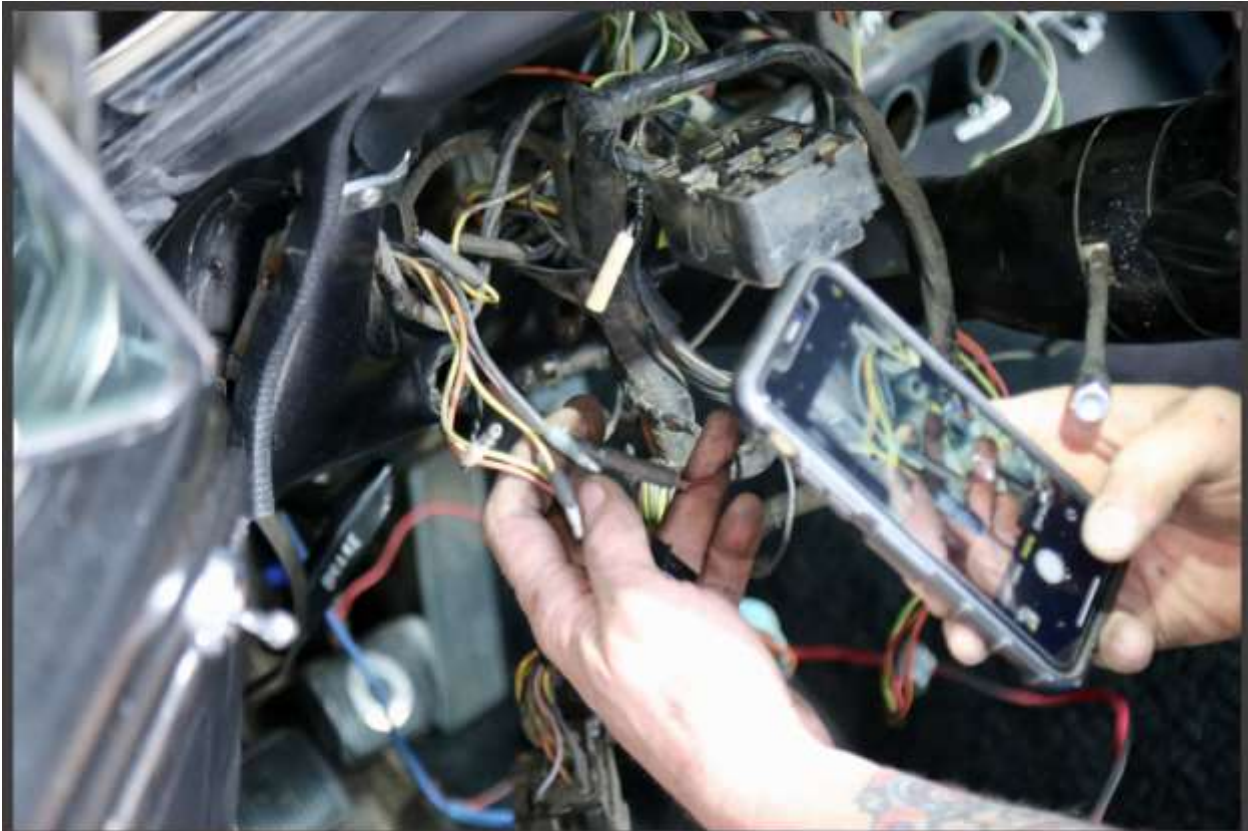
Barrett took cellphone photos of critical connections to help ensure correct hookups on the replacement harness.
