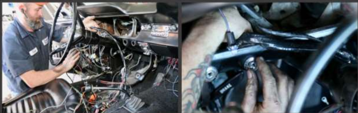
The new harness is carefully positioned over the steering to help facilitate the start of reconnecting the leads. Wires for the switches are identified and connected as the switches are installed.
