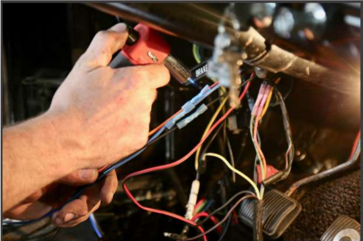
All the connections were finalized, and the insulations on some needed heat shrinking.
